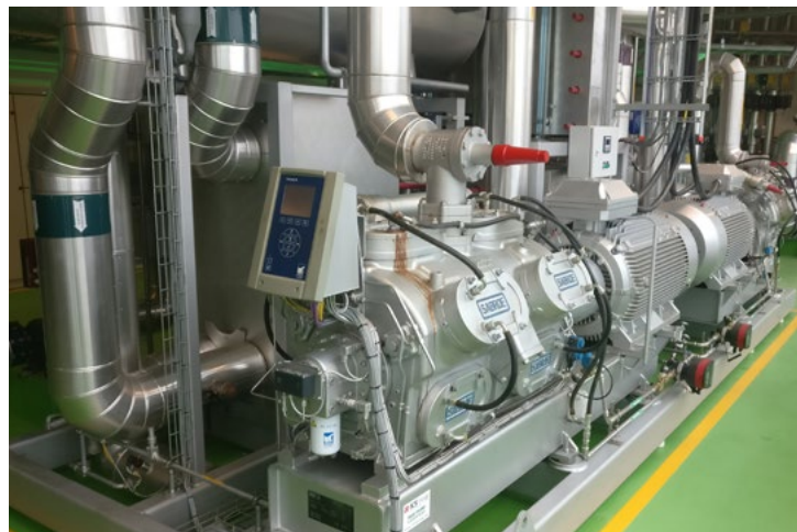
Heat pump for feeding waste heat into district heating networks, photo: 4ward Energy Research GmbH
