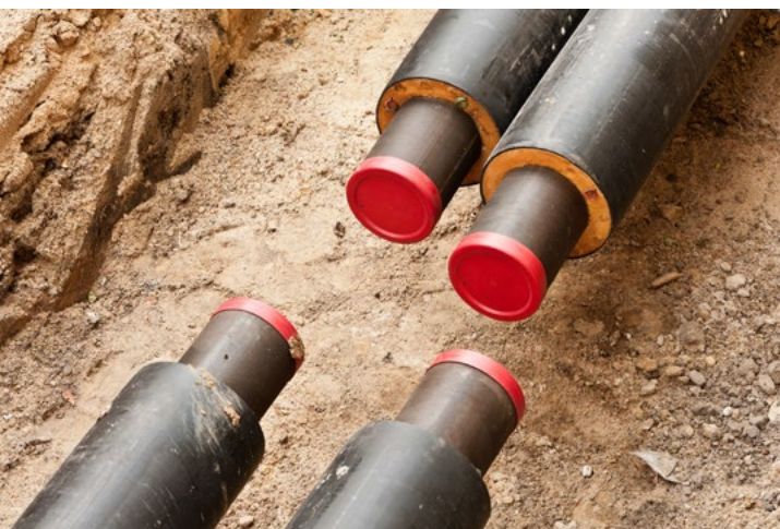
District heating pipes, photo: stock.adobe.com
