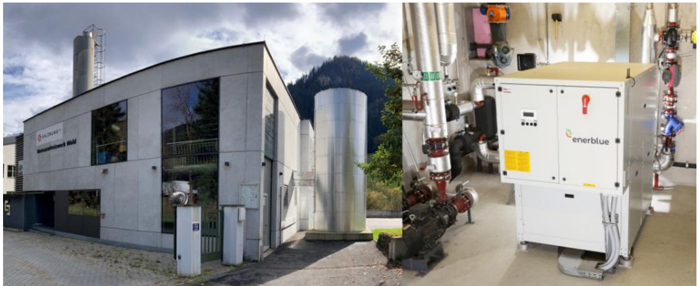
Figure 7: Left: DH plant with the 30 m 3 heat storage. Right: 250 kW th heat pump installed in the boiler house. Source: Klimafonds / Krobath
