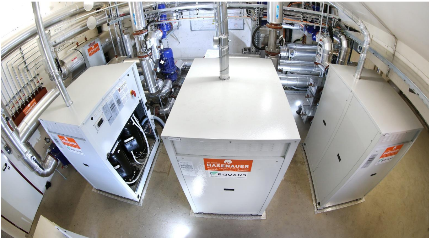
Figure 13: Cascading heat pump system (3 × 250 kW). Source: Klimafonds / Krobath
