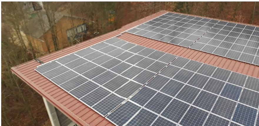
Figure 18: Installed PV collector field in Kreuzstetten. Source: Equans
