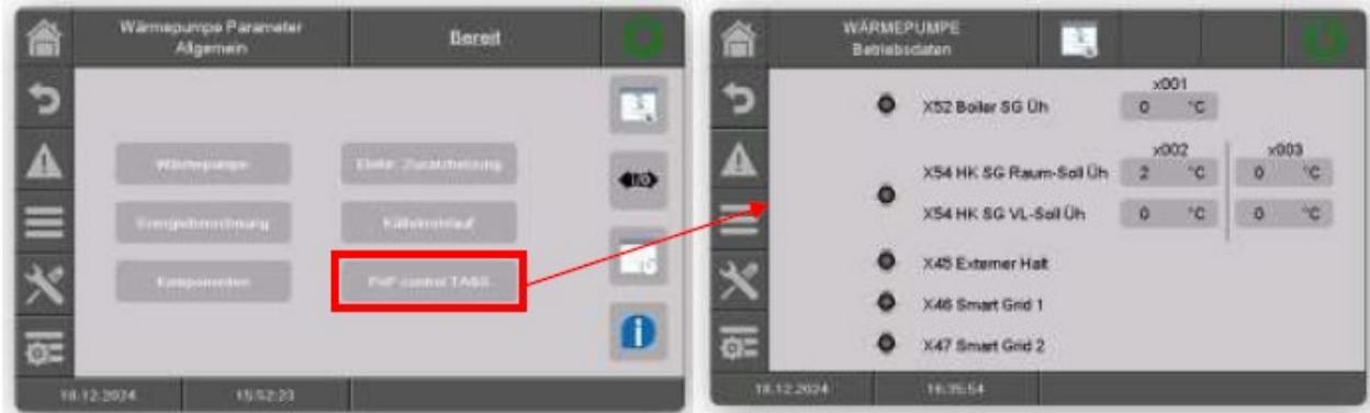
Figure 32: Software implementation of the PnP control logic in the HERZ heat pump controller (Source: ruvi e.U., 2024)
